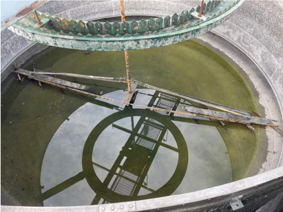
Clarifier #1: Steel Corrosion
