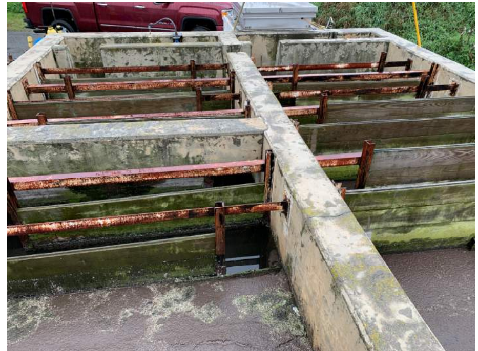
Chlorine Contact Tank – Undersized for Peak Flow
