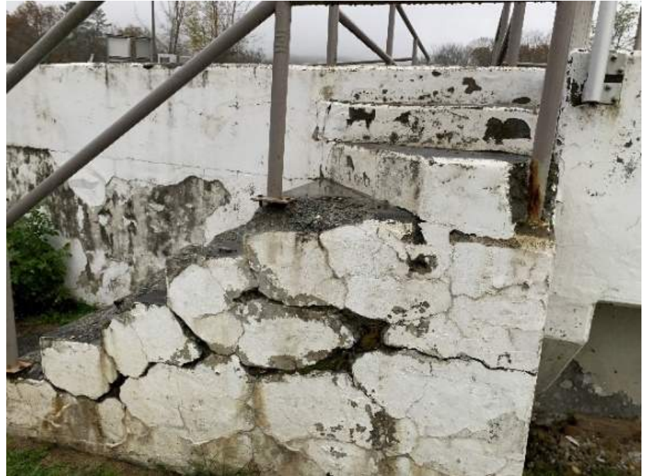
Aeration Tank: Concrete Defects
