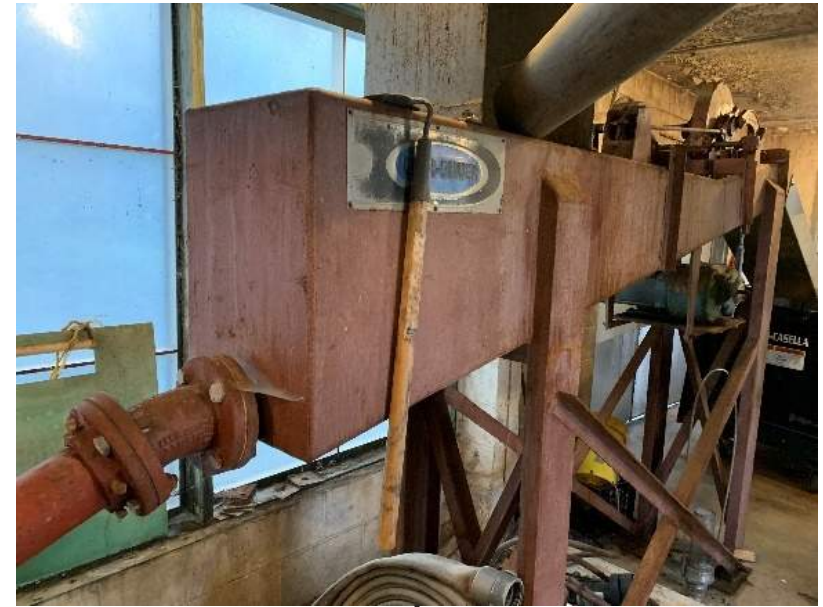
Grit Removal Equipment
